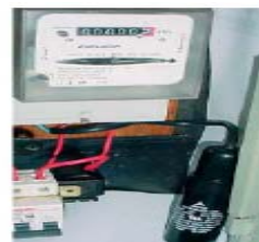
(a) Capacitor connected in meter box
